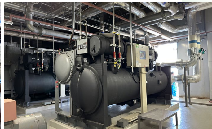
Refrigeration equipment with improved energy efficiency at the Noto Plant
